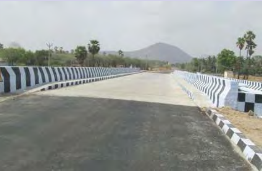
High Level Bridge at Veriyappur, Dindigul District inaugurated by the Hon'ble Chief Minister of Tamil Nadu on 20.06.2013
