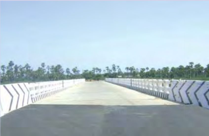
High Level Bridge at Mookaiyur in Ramnad District inaugurated by the Hon'ble Chief Minister of Tamil Nadu on 12-06-2014.
